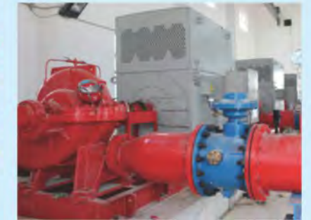
扬子石化电动消防泵 Sinopec Yangzi Petrochemical Electric Fire Pump
