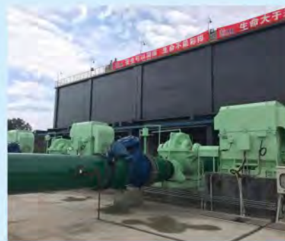
中石化茂名石化中开泵 Sinopec Maoming petrochemical Horizontal split case pump
