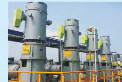
亨斯曼雨水泵 Huntsman rain water pump
