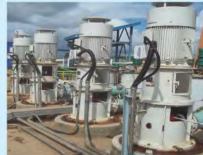
印尼南嘉电厂立式长轴海水泵 Namgyal Power Plant In Indonesia
