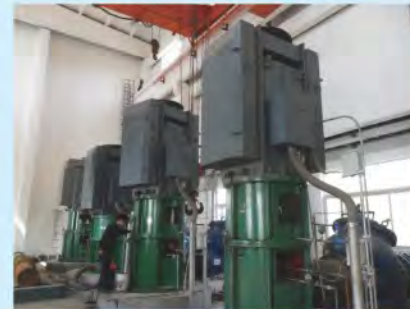
鲁阳电厂立式长轴泵(基础层以下长度23米) CNPC Luyang Power Plant (Length below foundation is 23m)
