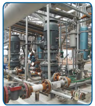
▲ CNOOC SHELL HUIZHOU REFINERY Flush Oil Pump Flow : 31m 3 /h Head: 175m Motor power: 37kW
